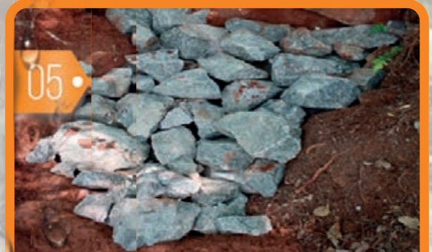
05. Large rocks are set inside the spring to prevent it from being smashed by animals that might walk on them, what could make water flow change its direction and consequently would make the spring useless.
