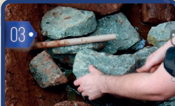
03. A second pipe is installed right above the first one in order to be connected with the farm house plumbing system;
