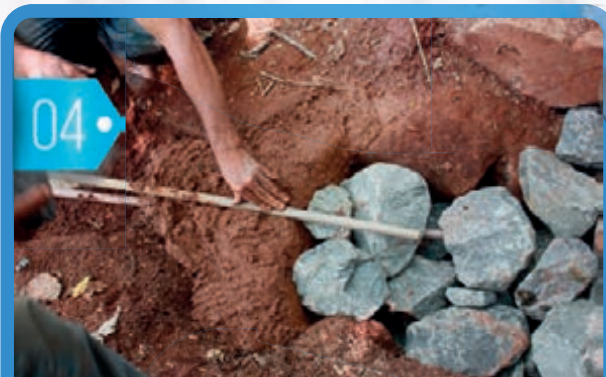
04. A last pipe is placed above the second one. Its function is to let excess water flow out so that it doesn't increase pressure inside the spring. This pipe has its outer protect with a fine net in order to prevent impurities to come into the spring.
